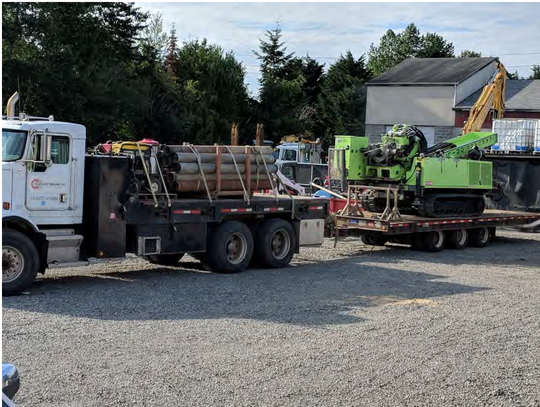
Photograph 4. Tracked drill rig and support vehicle similar to what may be used to drill borings other than LT-B4.
