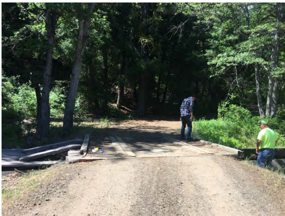
Photograph 6. The existing wooden bridge over the YTID canal may need to be strengthened to access LT-B4 (1,300 feet west of bridge).
