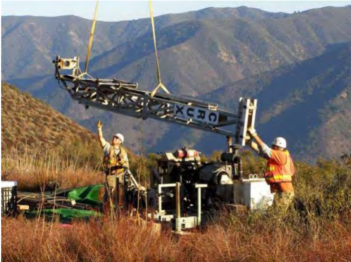
Photograph 1. Platform drill rig similar to what may be used to drill LT-B4.
