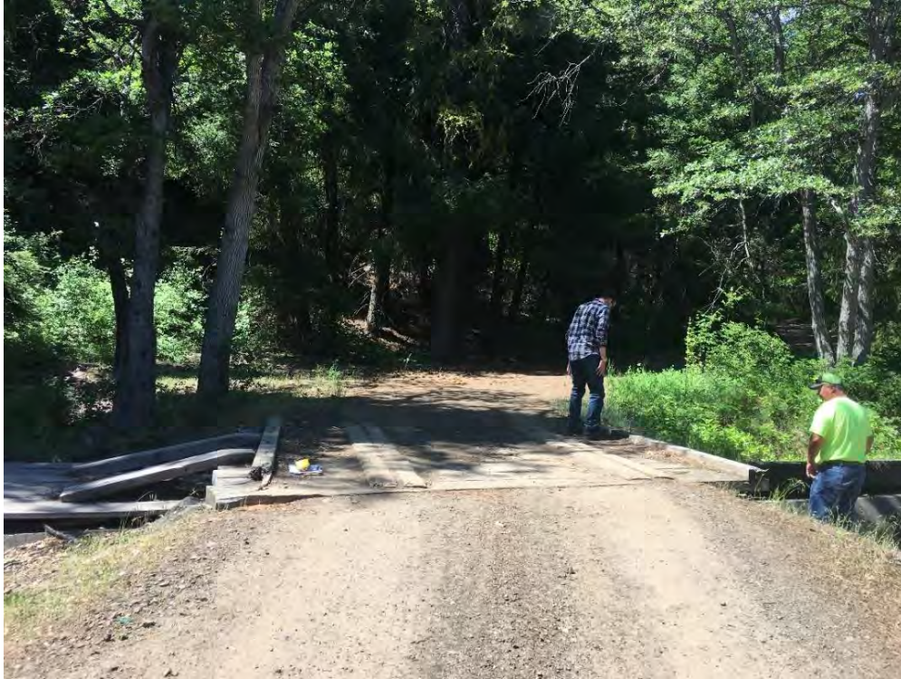
Photograph 14. Existing wooden bridge over YTID canal approximately 1,300 feet west of LT-B4. Bridge may need to be strengthened to access LT-B4.
