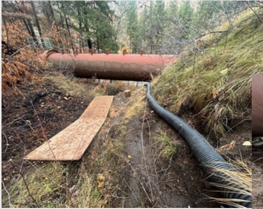
Before: Pipe bridge #1 with insufficient clearance for potential upcoming flooding & debris flow.
