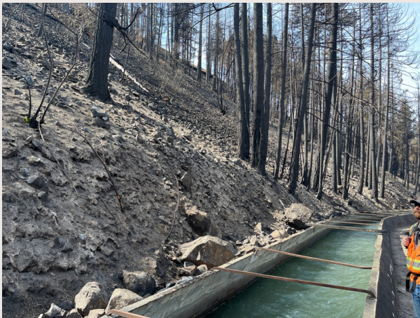
Before: Unstable burned terrain causing boulders to roll down the hill into the canal; conditions are anticipated to worsen in the spring due to lack of vegetation.
