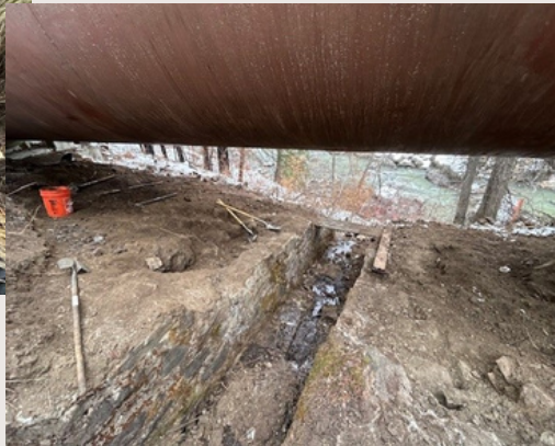
During Construction: Pipe Bridge #1 excavating an original drainage channel to increase clearance.
