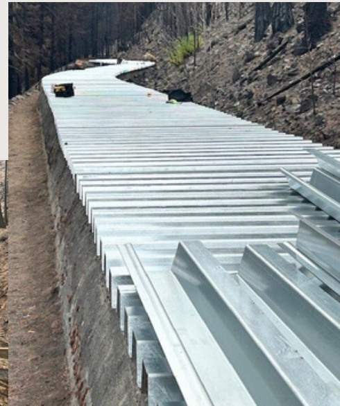
After: One section of the 6,000 linear feet of new cover installed. 10,000 feet of vulnerable area identified as highly vulnerable areas.
