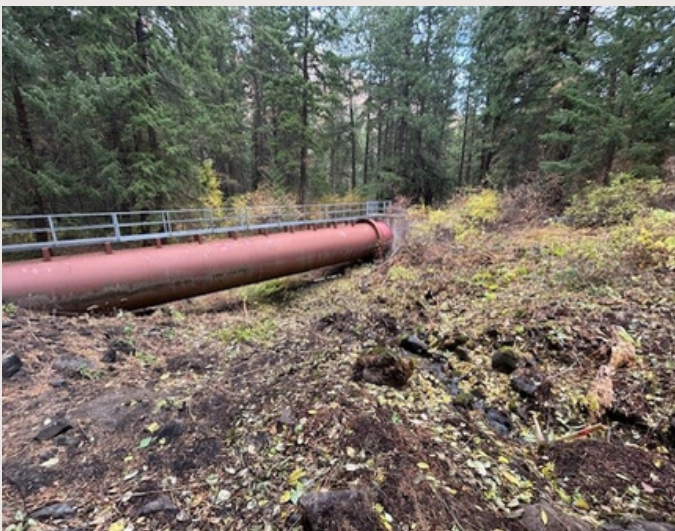
Before: Pipe bridge #2 upstream channel at risk and highly vulnerable to spring flooding and debris blockage.
