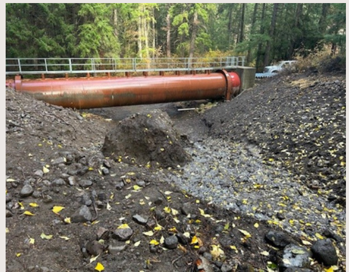
After: Pipe bridge #2 Significant material removed and channel open. (Note previously covered boulder).
