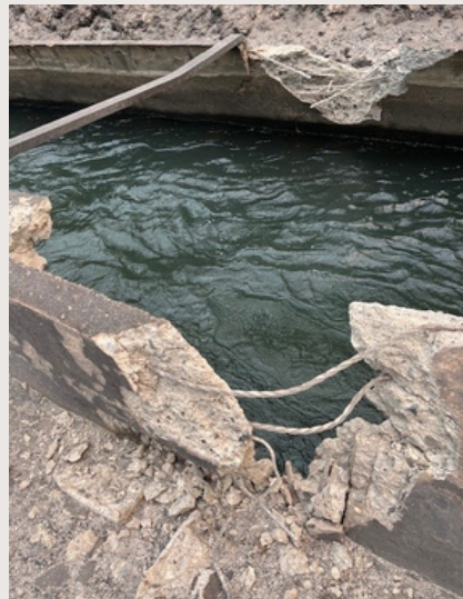
Boulder damage to canal.
