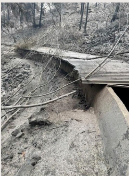
Before: All timber structures were lost in the fire, including cribbing meant to keep the weight of heavy cover off of the canal.
