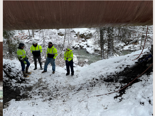
After: Pipe bridge #1 Now with adequate space to permit debris and water to pass underneath.
