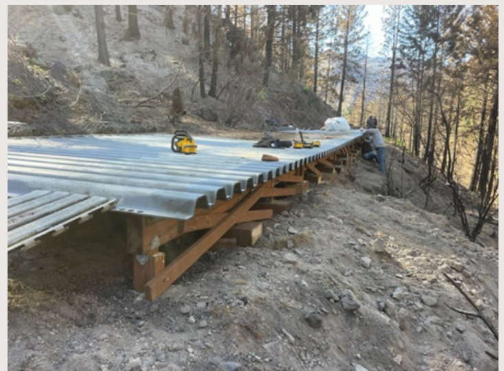
After: Timber cribbing re-installed at many locations to keep heavy decking from resting atop canal.
